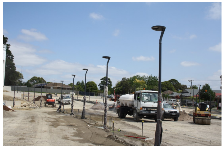
LED lights installed in the public car park.
