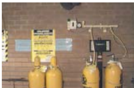
Figure 6 Chlorine gas, weight scales and regulator
