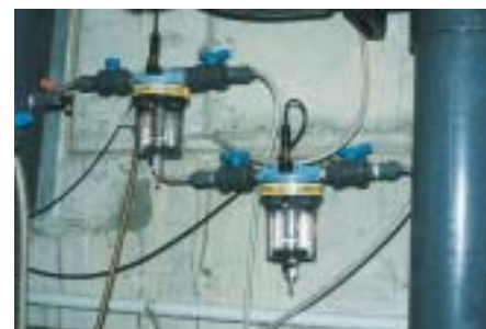
Figure 9 Pool water treatment with ozone and hypochlorite
