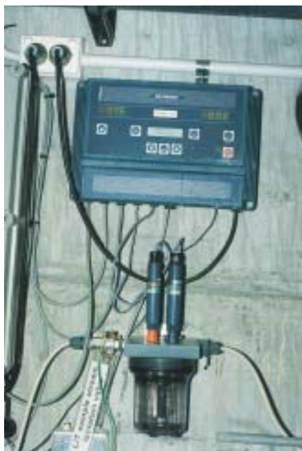
Figure 19 Chemical sensors installed in a side-stream loop
