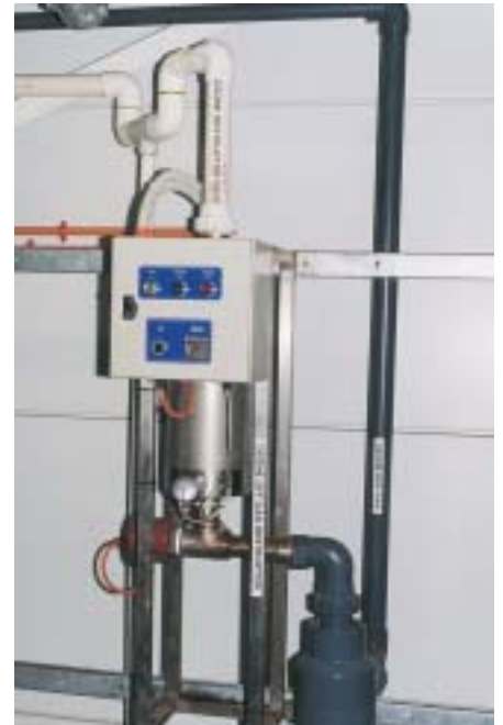
Figure 12 Ozone off-gas destructor
