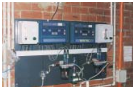
Figure 18 Pool control panel and chemical measuring station
