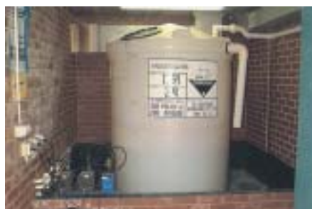
Figure 7 Bulk sodium hypochlorite container in bund
