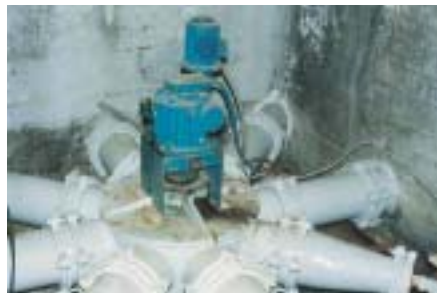
Figure 37 Multiport valve on a large, open gravity filter
