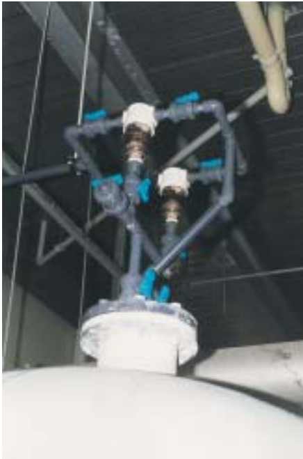
Figure 33 Filter off-gas bleed and collectors
