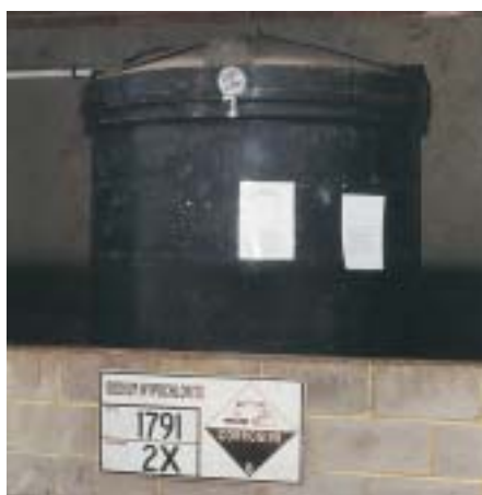
Figure 3 Hazchem signage for bulk dangerous goods
