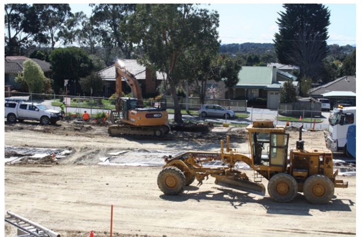
The heavy-duty plastic cell systems, to retain soil moisture for plant hydration, can be seen embedded in the car park medians.
