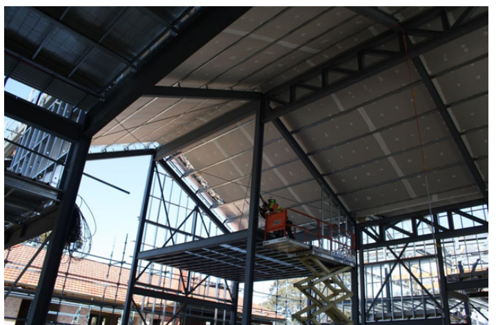
The central area of the building, which will be a large foyer, community library and relaxation space, has a pitched ceiling.
