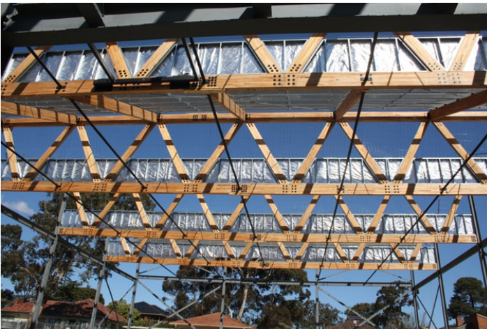
The stadium ceiling will have large exposed timber trusses forming a saw-tooth shape.
