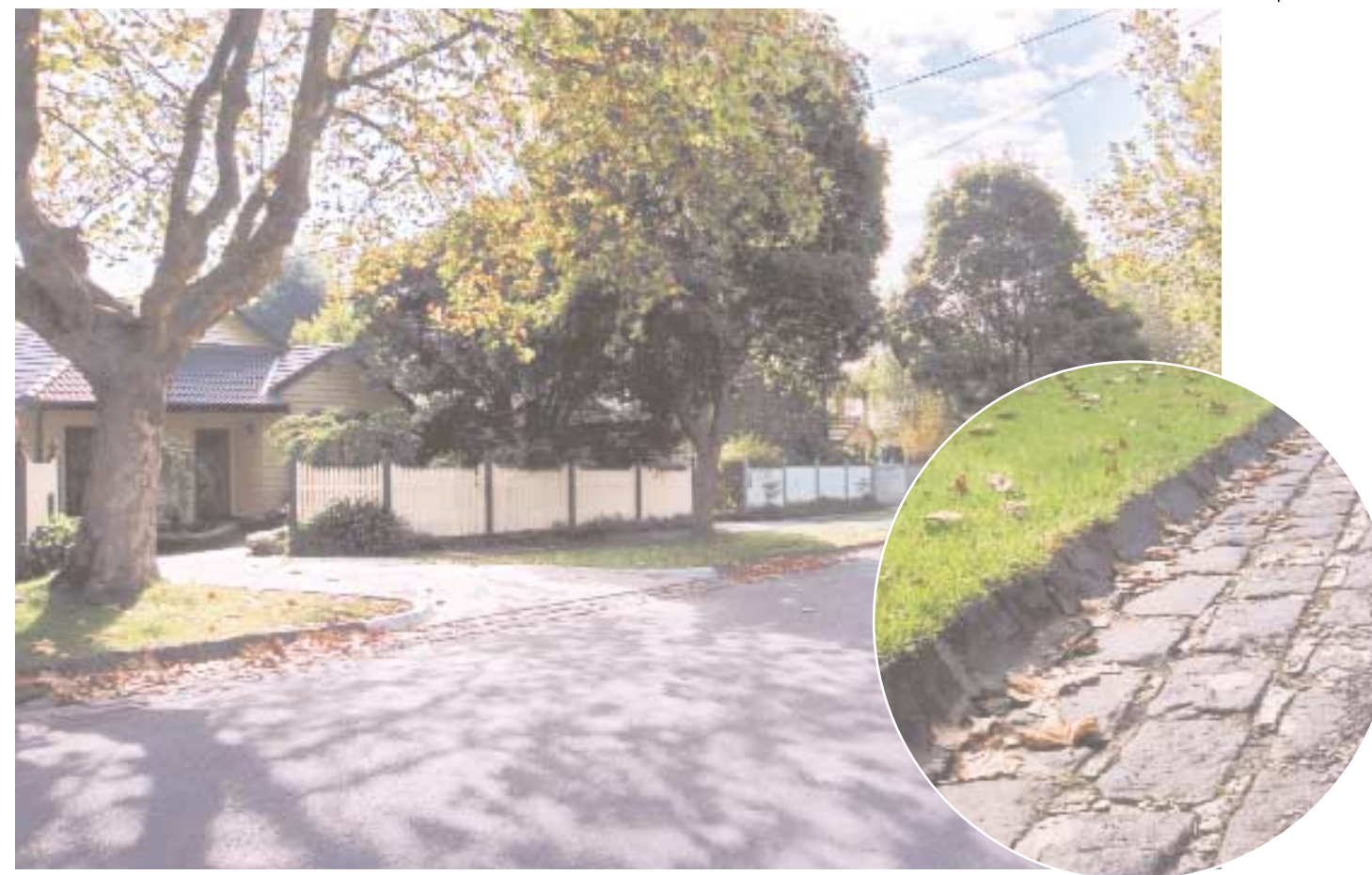
Photo 6. City of Whitehorse, 3 bluestone pitcher channel and kerb, Fellows Street, between Victoria Street and Ormond Avenue, Mitcham.
