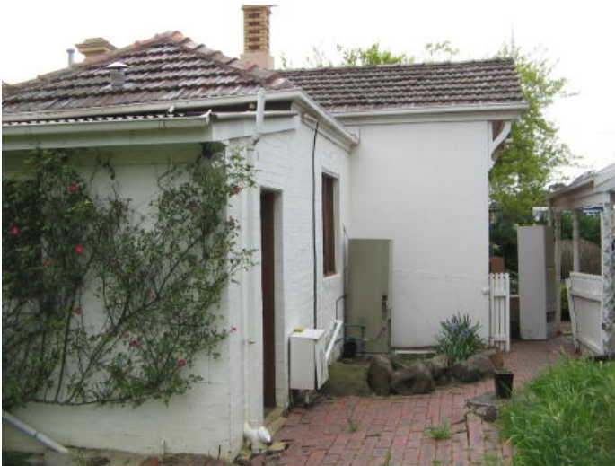
Rear of house south west corner showing gutter level & corrugated iron roof.
