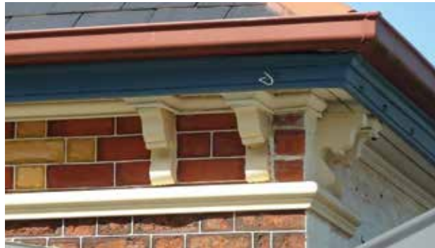
Repairs to damaged eaves and corbels (before photo)
