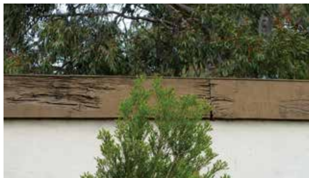
Replacement of rotting fascia board (before photo)
