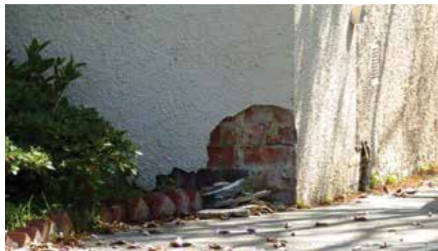
Repair to crumbling stucco render (before photo)
