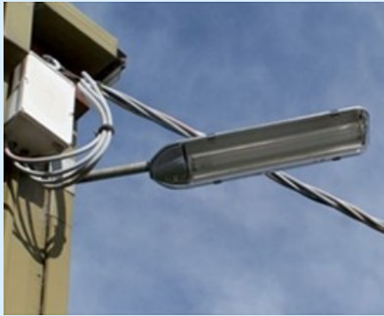
Figure 2: Example of T5 light installed during earlier phase of changeover
