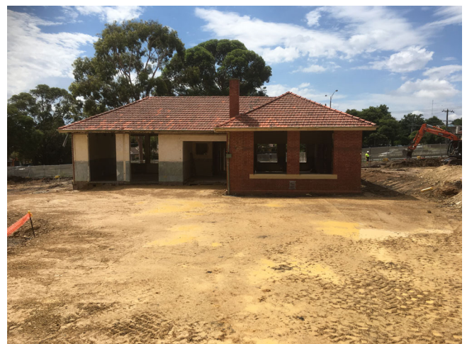
The heritage building has been cleaned up ready for restoration which will include strengthening and rendering of internal walls, installation of new windows and rectification of the façade.
