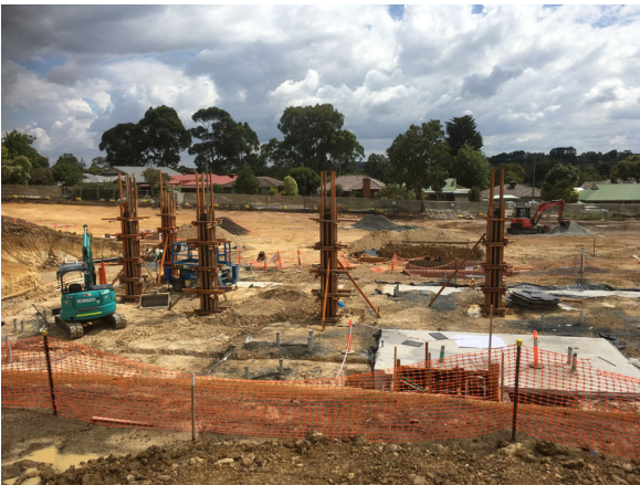
Columns are installed to support the lower ground level structure. The concreted elevator pit can be seen to the right in the foreground.
