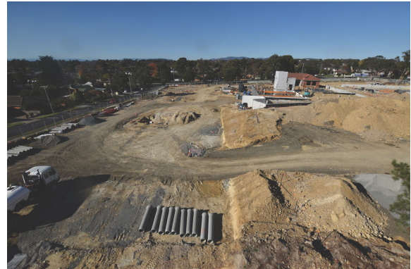
April 2019: Aerial view from Tunstall Park end shows trench works underway on the main car park with trucks taking away the excess soil. The beginnings of the retaining wall around the lower ground floor can be seen in front of the heritage building in the background.
