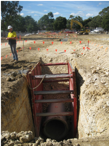
April 2019: Large storm water pipes are installed under the main car park which will accommodate 200+ cars.
