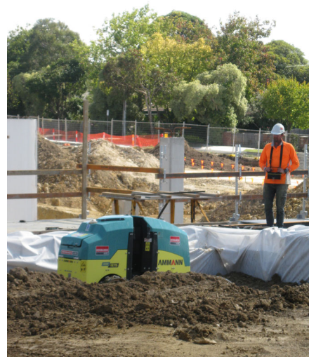
April 2019: A remote-controlled mini compacting machine is able to access tight spaces to compact down the soil.
