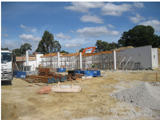
April 2019: A concrete retaining wall is being installed around the lower ground floor.
